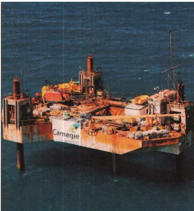
The jack-up rig Carnegie Wave Energy is using to build its wave energy facility west of Garden Island.
